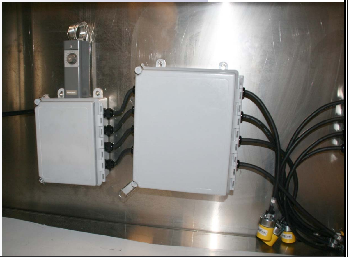
Illustration 2.B- Breaker Box, Distribution Block Box, Rear Distribution Panel
